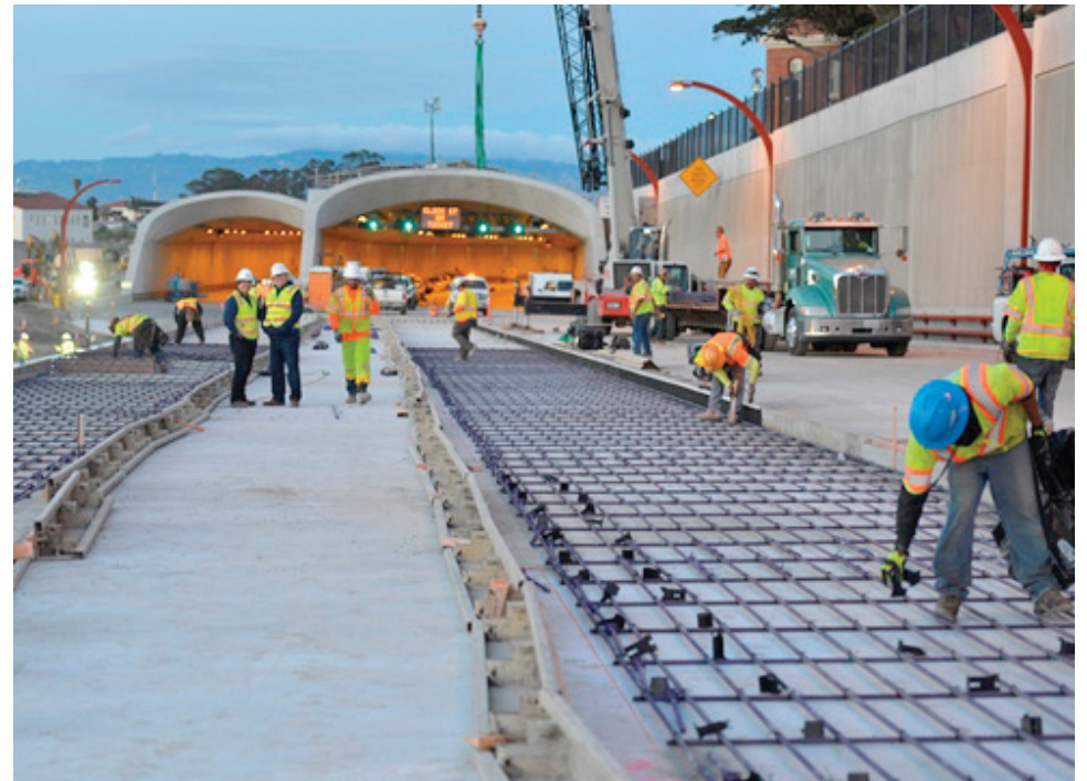
Crews labored 40 hours nonstop during a recent road closure to transfer traffic to new structures. The roadway was reopened eight hours ahead of schedule. Photo courtesy of Byron Lim
